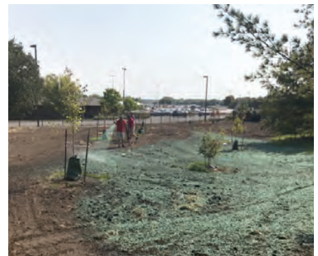
Using the hydroseeder at Reiman Gardens when seeding area that was finished with construction.
