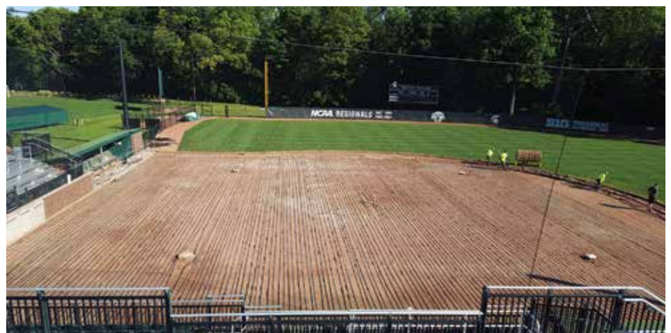
New field heating system on softball field.
