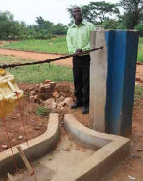
Drainage under hand-washing station.
