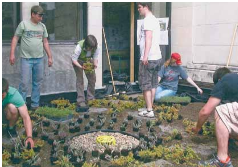
Horticulture Hall green roof installation on May 6, 2011, a major impetus for the idea of a green roof course.
